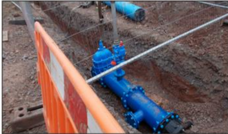
Watermain diversion carried out within existing works with help from CR Civil Engineering
